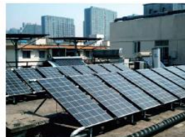
Hangzhou Energy Institute Commercial Solar System 10kW
