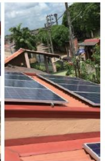
Sri Lanka Residential Solar System 5kW
