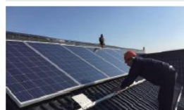
Quzhou Shiliang Residential Solar System 5kW
