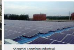
Shanghai Kangshun Industrial Solar Systems 1.2MW
