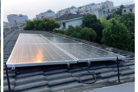
Quzhou Villa Residential Solar System 2kW
